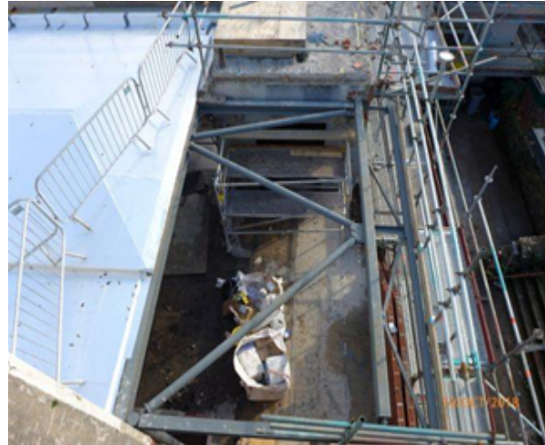
Looking South: New Roof over First Floor Offices & RPM Studio (NB: Work in Progress - roof framing at the West end remains to be completed).
