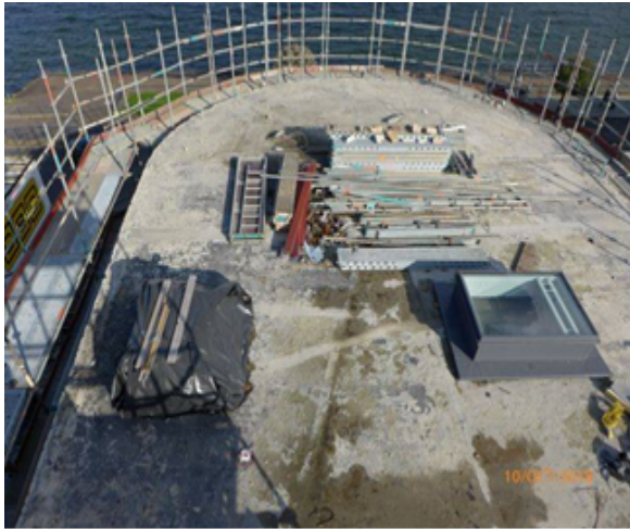
Looking East (facing Argyle St): Canopy Roof over new First Floor Exhibition/Function Area.
