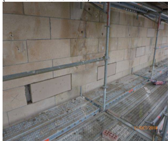
East Elevation (Argyle St.) – NB: Work in Progress: defective cast stonework replacement with new stone).
