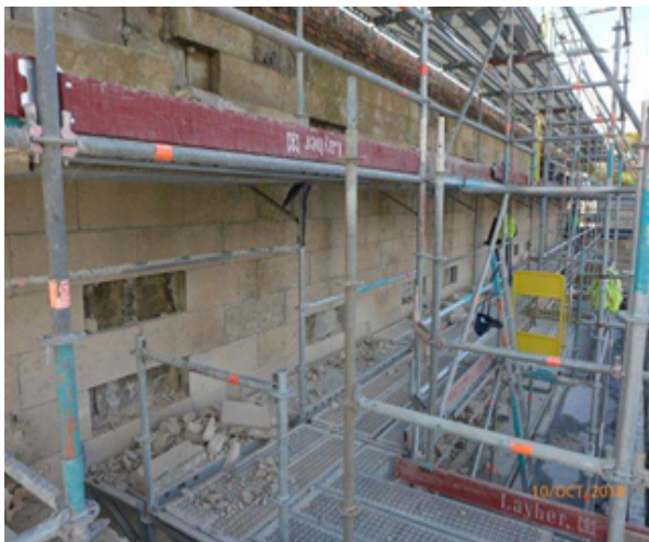
East Elevation (Argyle St.) – (NB: Work in Progress: defective cast stonework removal in progress).
